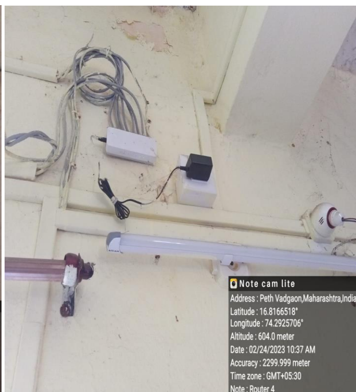
Router No. 4 Staff Room
