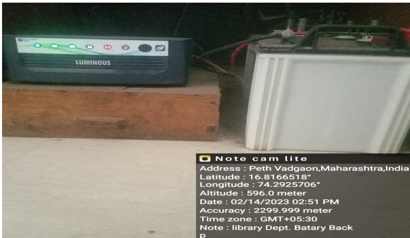
Battery Backup System – Library Department
